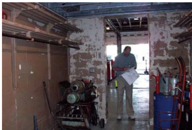
Drying tube ducts ran non-stop for months in the inside of Veterans Memorial/City Hall to dry out the interior.
